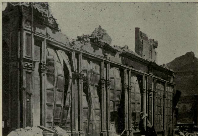
FIG. 117. — Plate-iron Shutters in San Francisco Conflagration.
